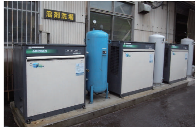
Manufacturing plant: SMS8ESD x 1, SMS11ESD x 2
